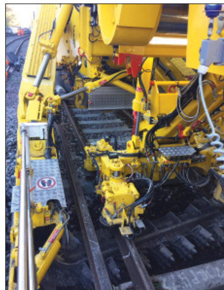
Left and above: The RM 900 ballast cleaner making its first cut on the section of third rail fitted track at High Marnham.
